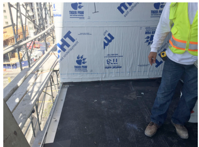
Photograph 7: Drip Edge and Drainage Matt —The water resistive barrier (WRB) is lapped over the membrane waterproofing. A drainage mat is in place as is the drip edge at the balcony edge.
