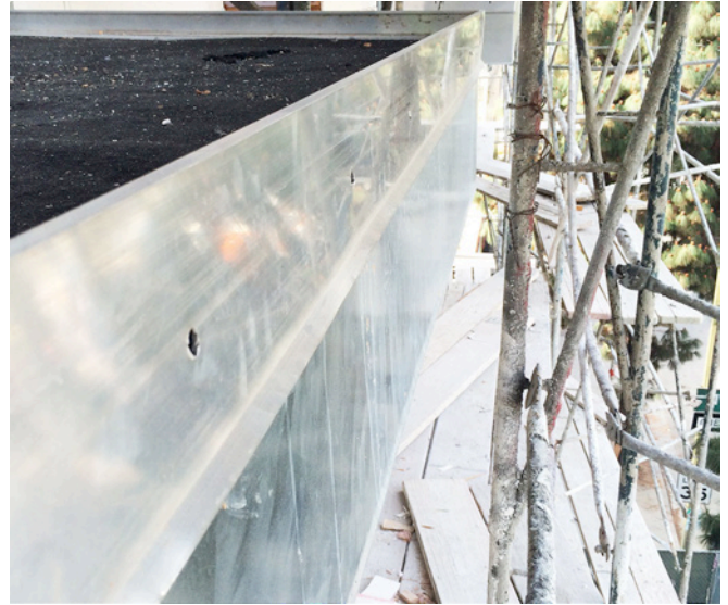
Photograph 9: Two Drip Edges —The upper drip edge sheds water flowing over the edge of the concrete topping. The lower drip edge sheds water from the drainage mat gap on the top of the waterproofing membrane under the concrete topping. This two-stage drip edge approach is recommended to deal with any minerals carried in solution in drain water exiting the drainage mat gap.
