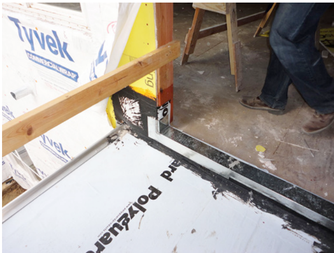
Photograph 4: Membrane Waterproofing —Additional metal flashing is installed over the waterproofing that is stripped into the pan flashed balcony door opening. This additional metal flashing protects the membrane waterproofing at the door opening.
