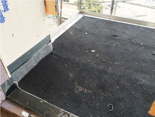
Photograph 8: More Drainage Matt —The vertical top edge of the perimeter balcony deck waterproofing membrane is yet to be stripped into the exterior wall sheathing with mastic.
